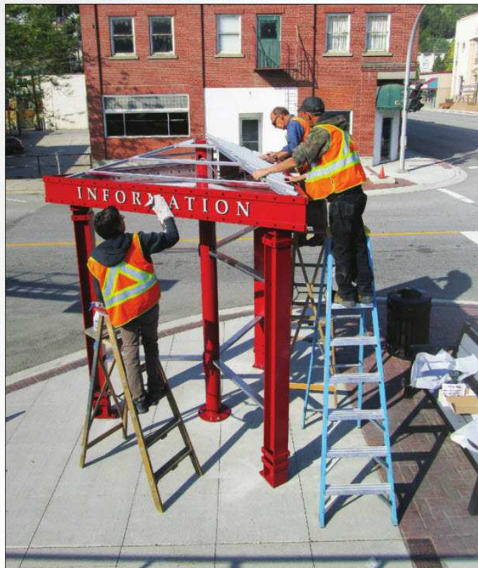
A crew from Best Canadian Lighting and Signs in Vernon was assembling a new information kiosk at the corner of Victoria St. and Cedar Ave., in downtown Trail on Tuesday morning. The kiosk will feature maps, event listings and city projects. See story on Page 3.
